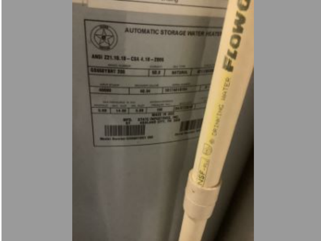
Garage Water Heater Water heater label
