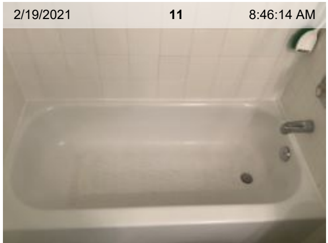
Tub/Fixture | Base of Tub
