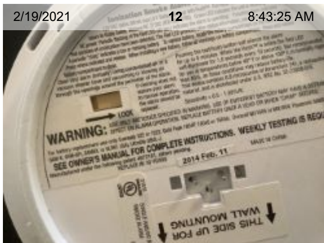
Wired Smoke Alarm (mfd 2/2014) | Smoke test: Passed | Close-up of printed manufacture date
