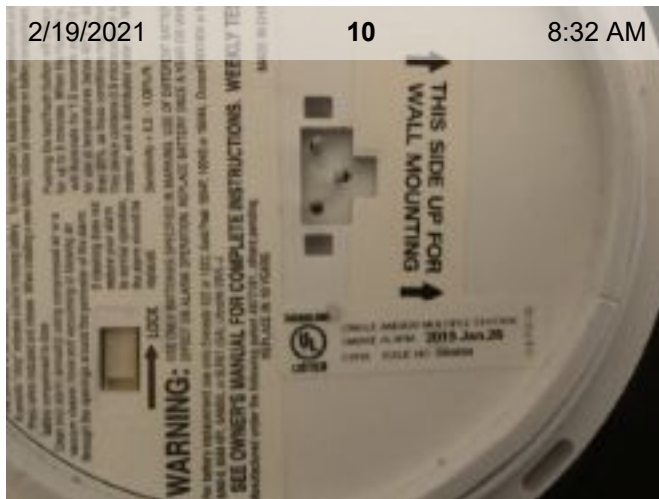
Wired Smoke Alarm (mfd 1/2015) | Smoke test: Passed | Close-up of printed manufacture date
