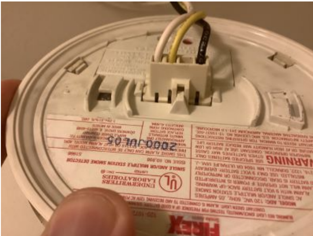
Kitchen Smoke Alarm Close-up of printed manufacture date (typically on back of alarm) Connector does not match alarms in technicians inventory
