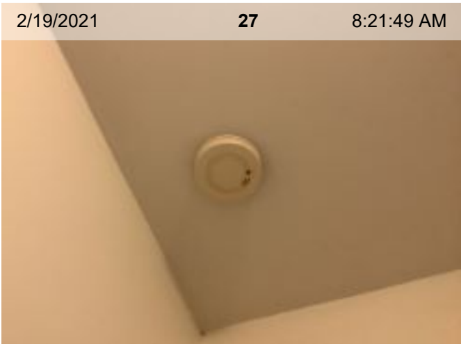
Wired Smoke Alarm (mfd 7/2000) | Smoke test: Failed | >10 yrs old | Alarm in place (on ceiling or wall)
