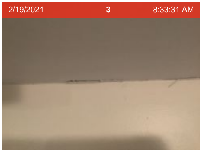
Ceiling | Slight separation of wall and ceiling (see closeup).
