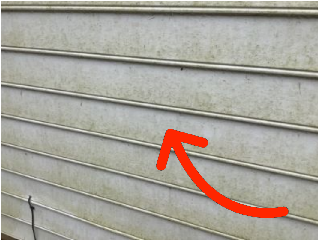
Front Exterior Walls/Siding/Trim Siding is discolored
