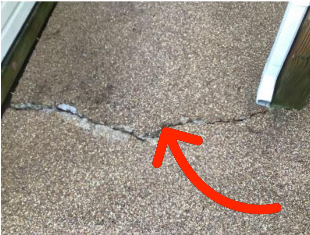
Rear Exterior Porch/Patio/Deck Crack.
