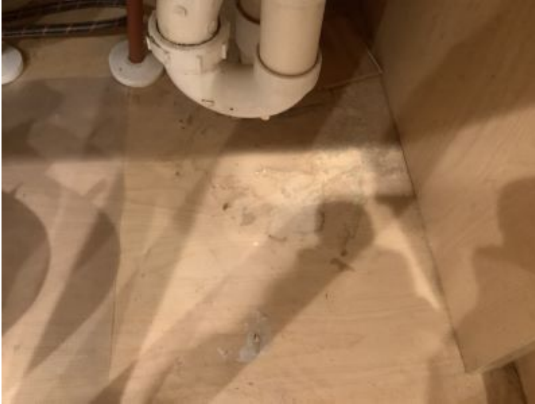
Kitchen Cabinet Under Sink Damage to base of cabinet
