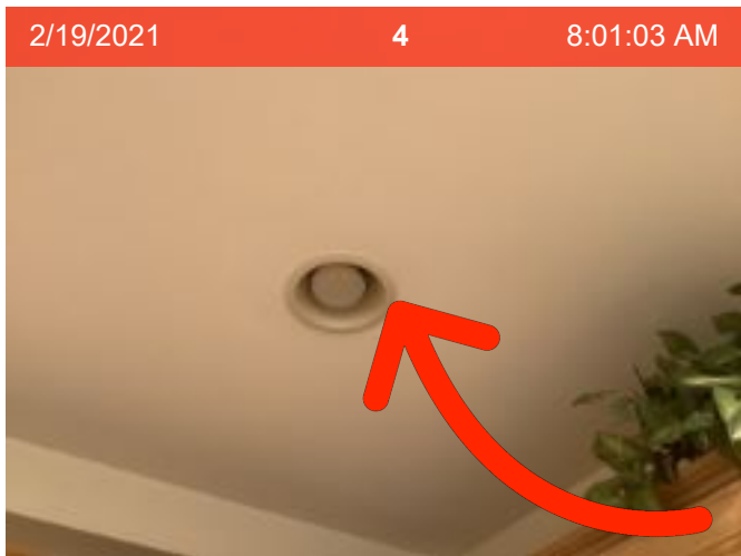
Light Fixtures | Light did not turn on. |
