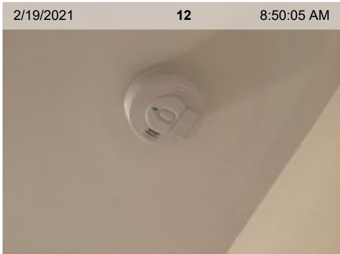
Wired Smoke Alarm (mfd 2/2014) | Smoke test: Passed | Alarm in place (on ceiling or wall)
