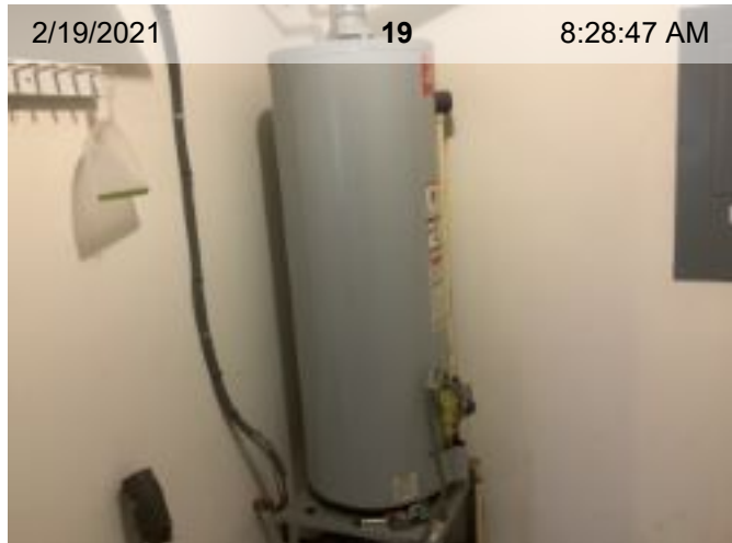
Gas Water Heater | >10 yrs old | State | Water heater (with expansion tank if present)
