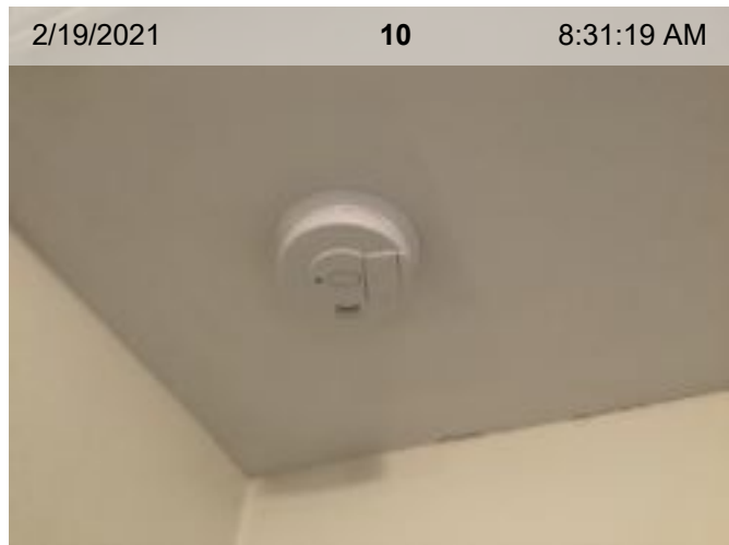
Wired Smoke Alarm (mfd 1/2015) | Smoke test: Passed | Alarm in place (on ceiling or wall)
