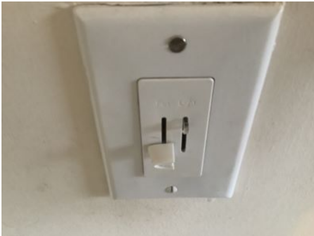
Bedroom 1 Outlet/Switch Covers Knob missing
