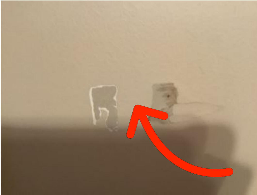
Bedroom 3 Walls/Paint Scratches on the wall
