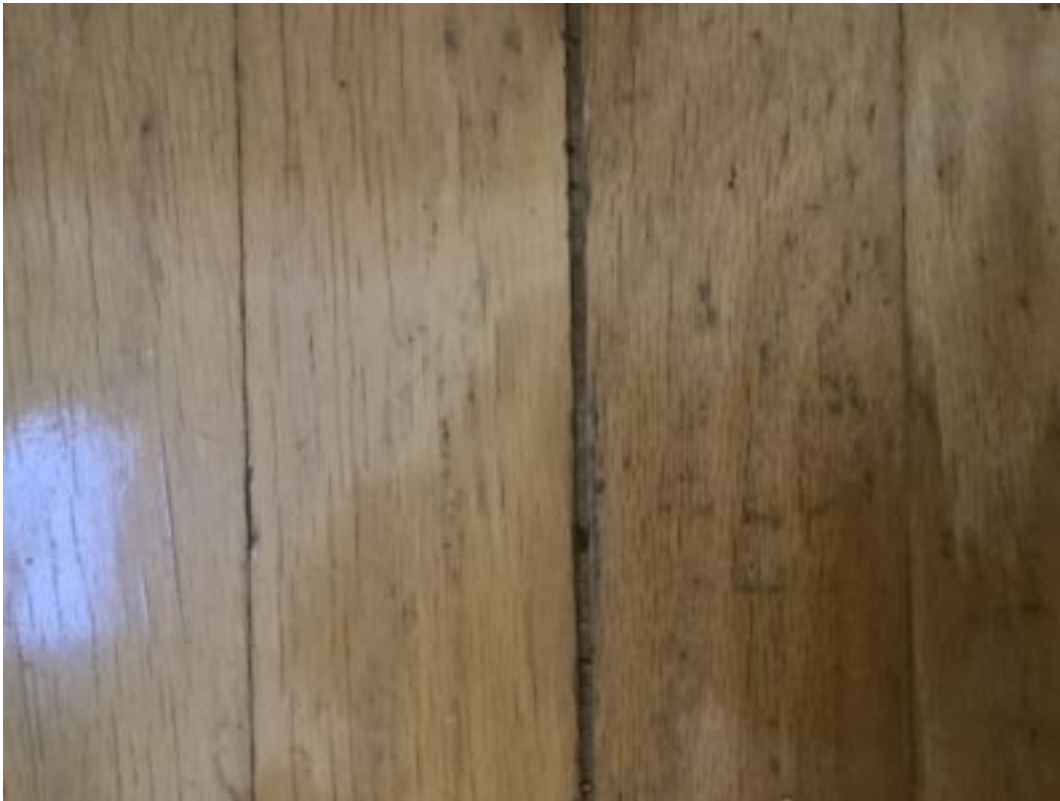
Entry Floors Gap in flooring.
