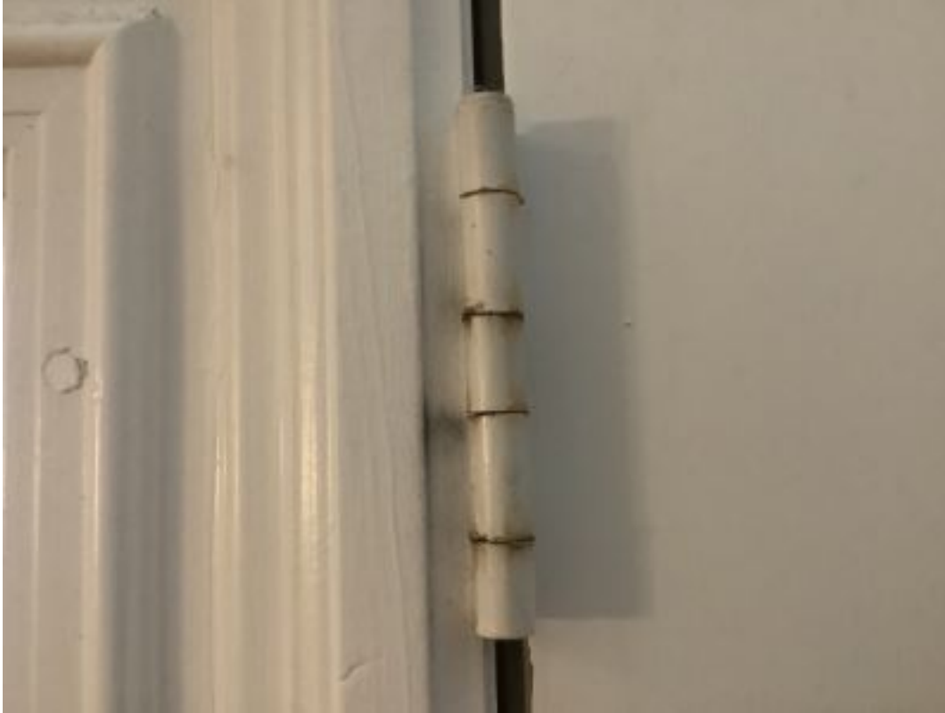
Entry Door Stop Doorstop missing, area not appropriate for wall plate or standard doorstop
