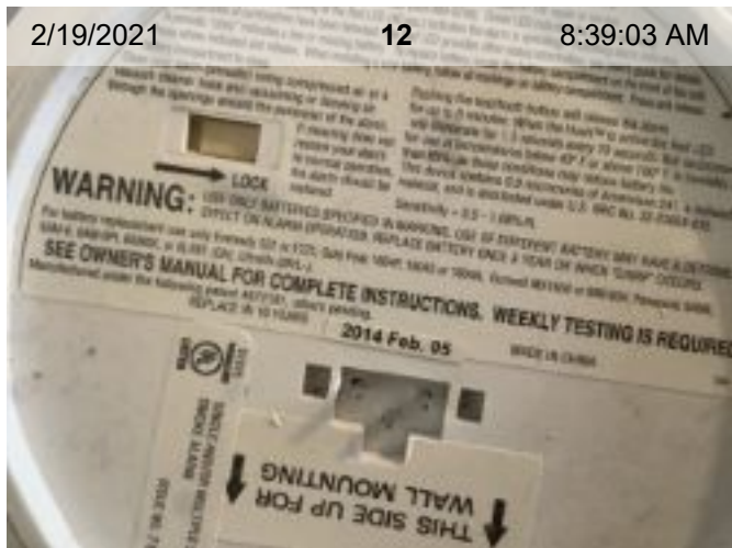
Wired Smoke Alarm (mfd 2/2014) | Smoke test: Passed | Close-up of printed manufacture date
