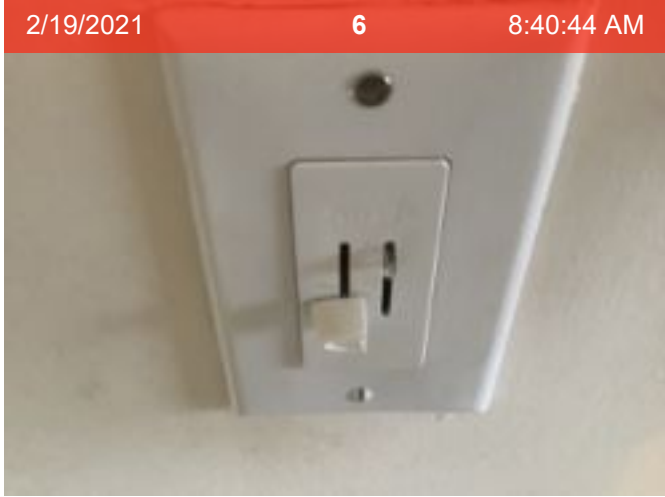
Outlet/Switch Covers | Knob missing
