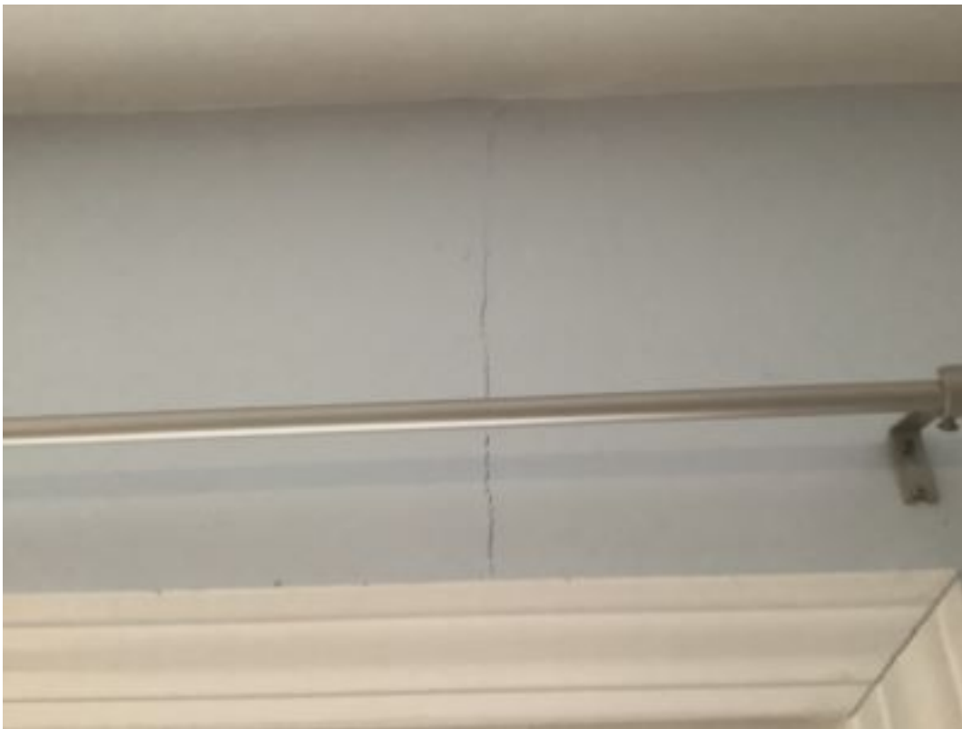
Bedroom 2 Walls/Paint Cracks in texture
