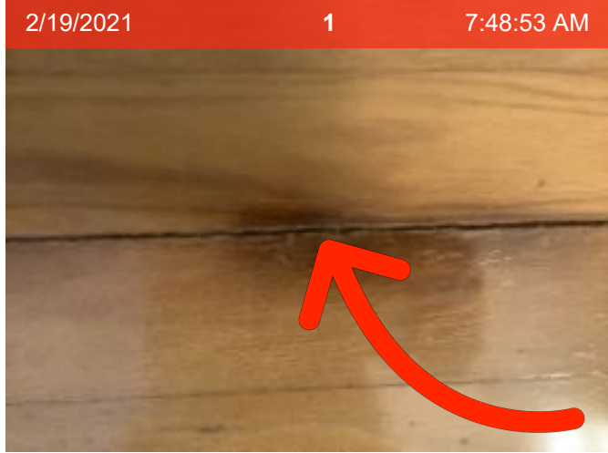
Floors | Discoloration and gap.
