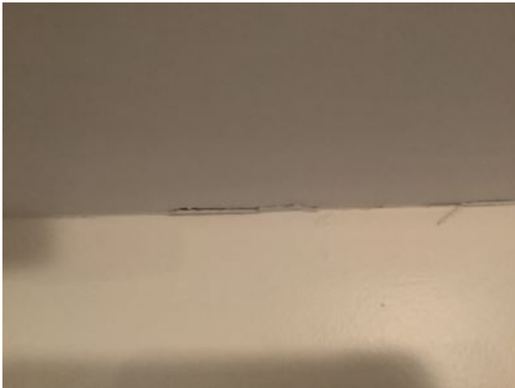
Hallway/Stairway Ceiling Slight separation of wall and ceiling (see closeup).
