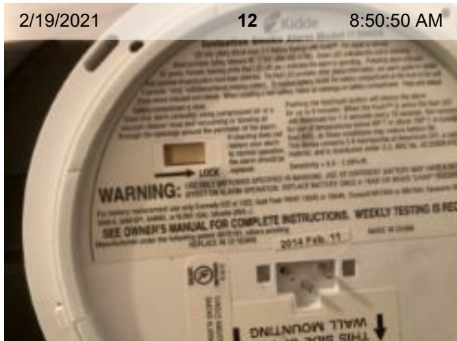
Wired Smoke Alarm (mfd 2/2014) | Smoke test: Passed | Close-up of printed manufacture date
