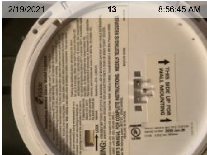
Wired Smoke Alarm (mfd 1/2015) | Smoke test: Passed | Close-up of printed manufacture date
