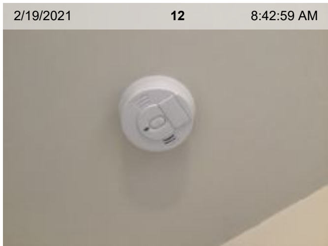
Wired Smoke Alarm (mfd 2/2014) | Smoke test: Passed | Alarm in place (on ceiling or wall)
