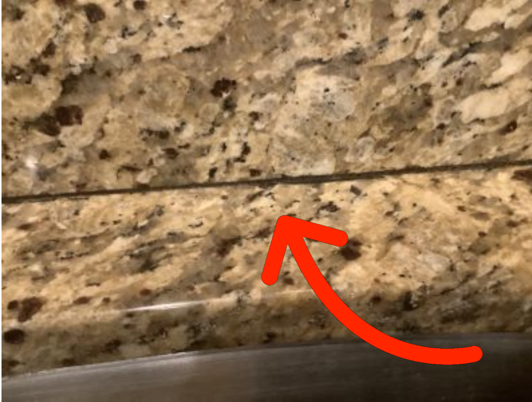
Kitchen Counter Top/Back Splash Caulk is discolored where counter meets the wall.
