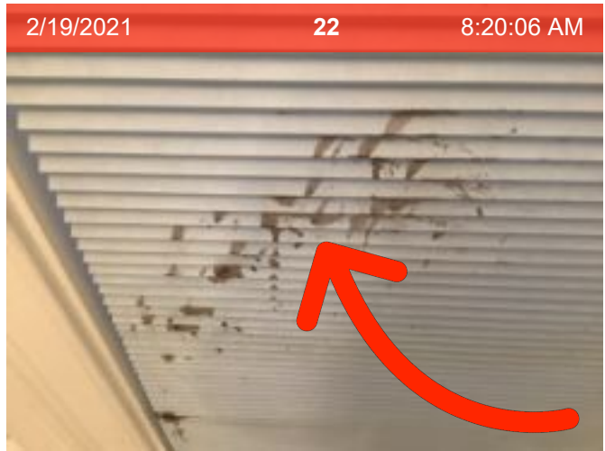
Blinds/Drapes | Stain on blinds
