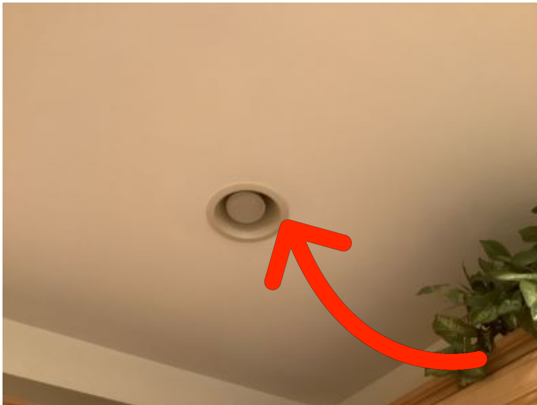
Kitchen Light Fixtures Light did not turn on.
