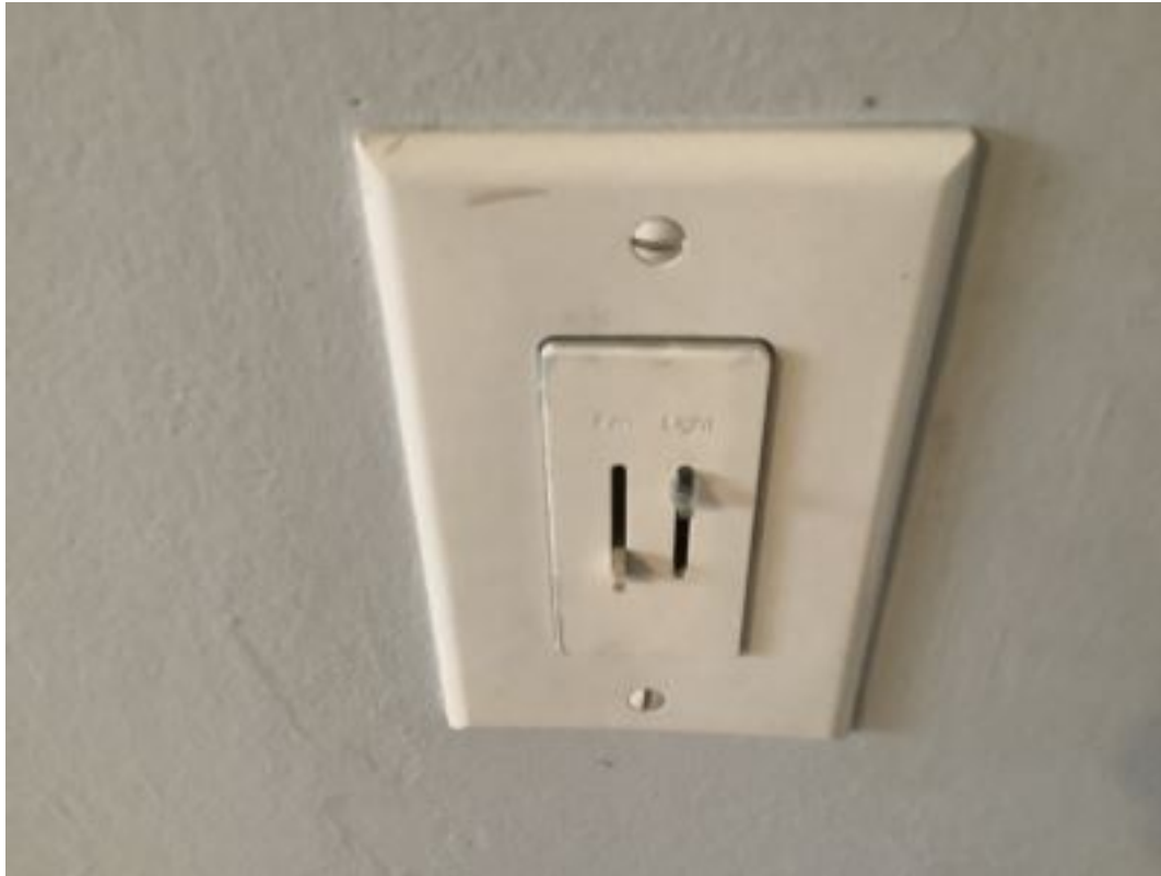
Bedroom 5 Outlet/Switch Covers Knobs missing.
