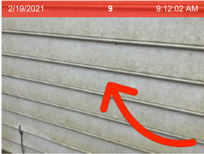
Walls/Siding/Trim | Siding is discolored
