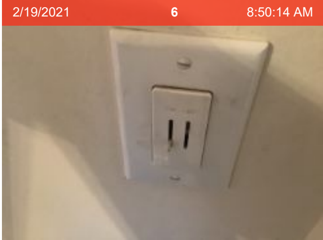
Outlet/Switch Covers | Knobs missing
