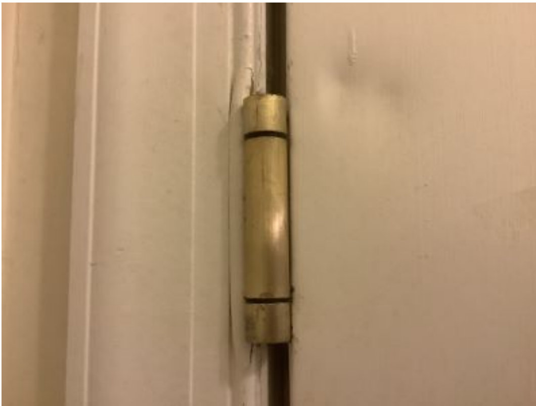
Garage Door Stop Doorstop missing, area not appropriate for wall plate or standard doorstop
