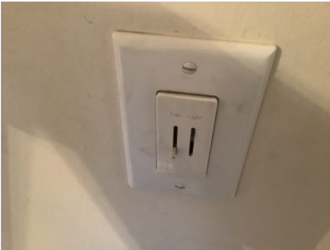
Bedroom 4 Outlet/Switch Covers Knobs missing
