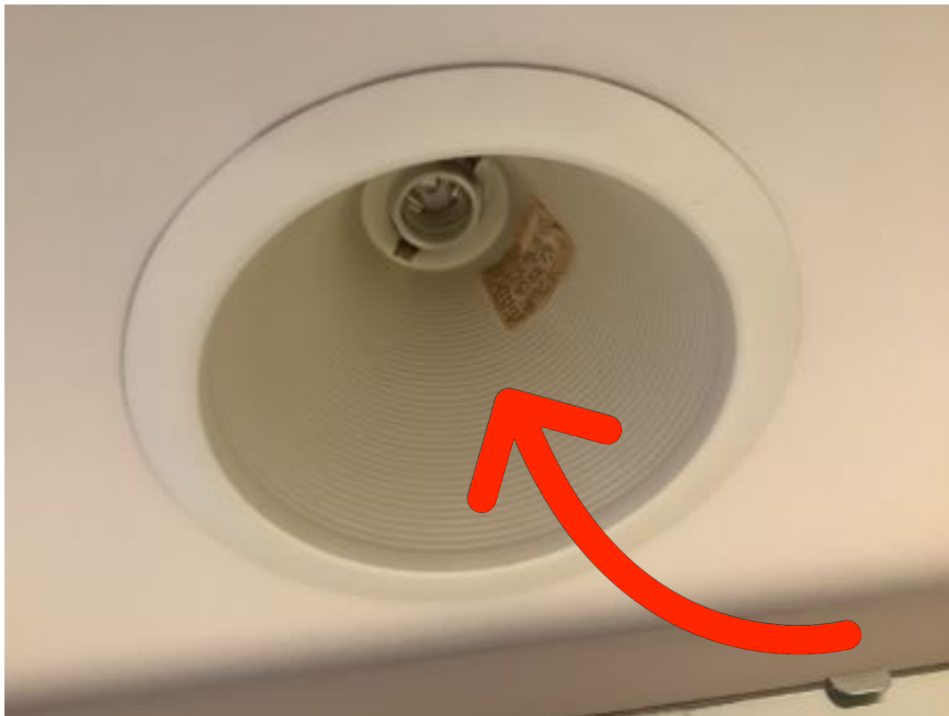
Bathroom 3 Light Fixtures Bulb is missing
