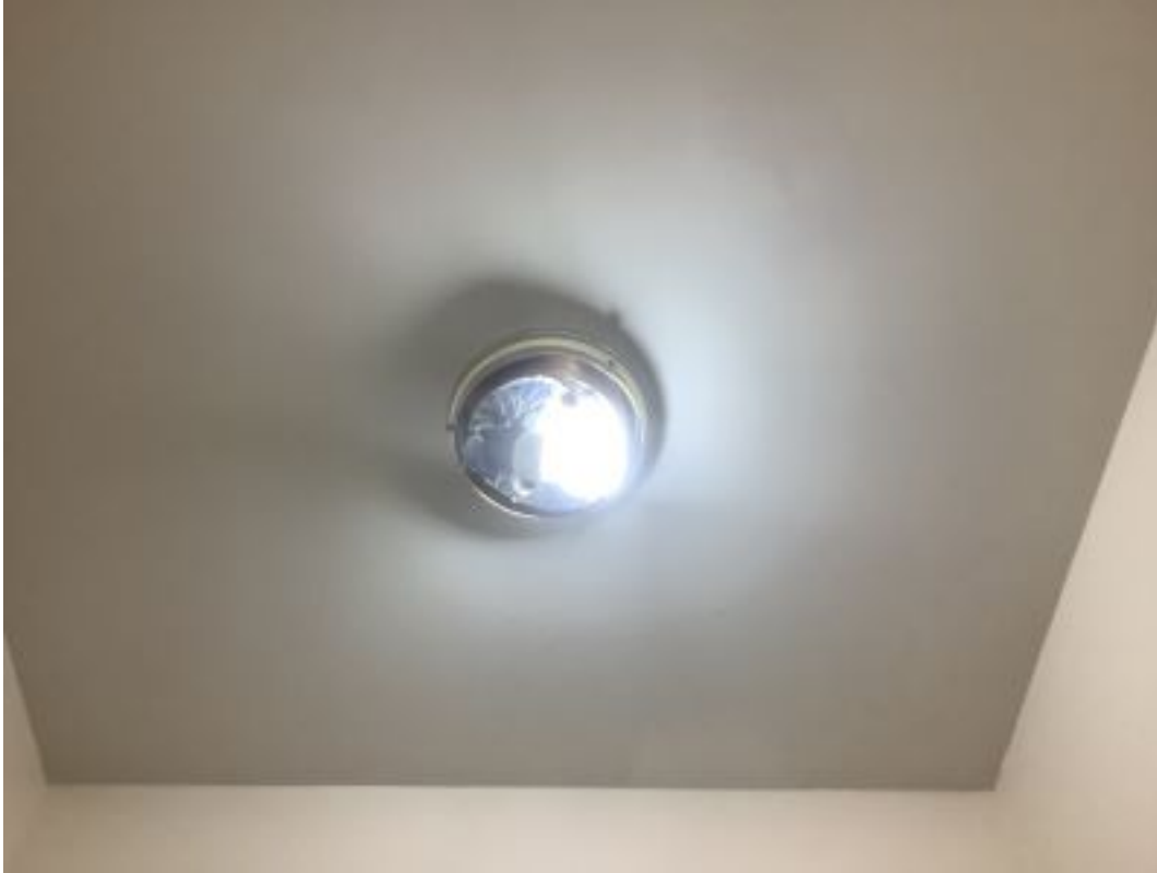
Living Room Light Fixtures Missing globe
