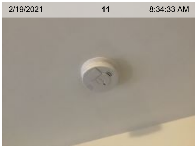
Wired Smoke Alarm (mfd 1/2015) | Smoke test: Passed | Alarm in place (on ceiling or wall)
