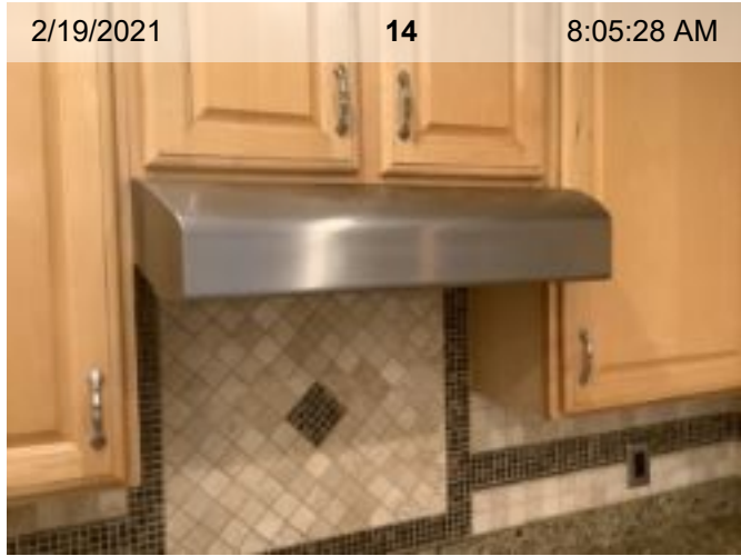
2/19/2021 14 8:05:28 AM Exhaust Fan
