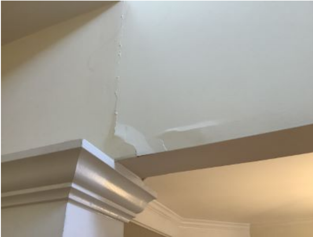
Entry Walls/Paint Cracks in texture
