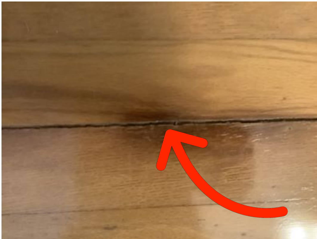
Dining Room Floors Discoloration and gap.
