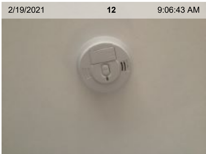
Wired Smoke Alarm (mfd 2/2014) | Smoke test: Passed | Alarm in place (on ceiling or wall)
