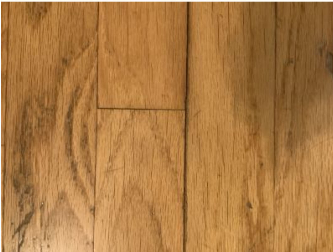
Living Room Floors Gap in flooring.
