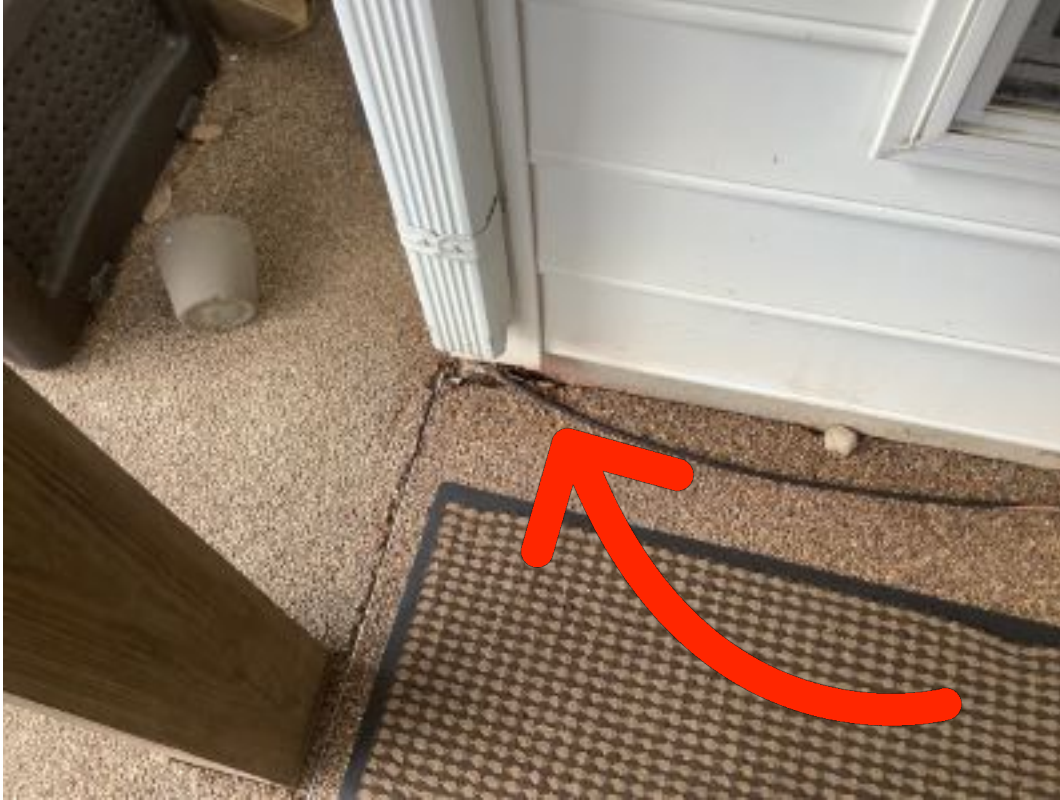
Rear Exterior Downspout/Splash Blocks Lower elbow and splash block missing
