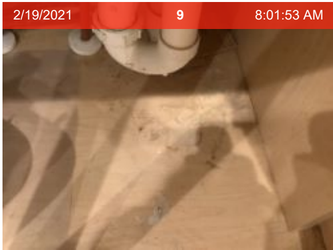
Cabinet Under Sink | Damage to base of cabinet
