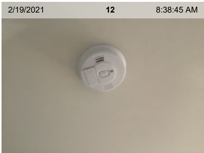
Wired Smoke Alarm (mfd 2/2014) | Smoke test: Passed | Alarm in place (on ceiling or wall)
