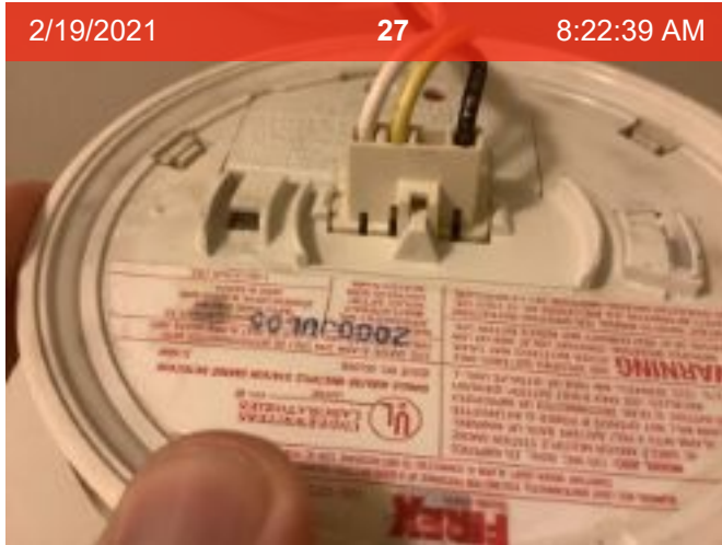
Wired Smoke Alarm (mfd 7/2000) | Smoke test: Failed | >10 yrs old | Close-up of printed manufacture date
