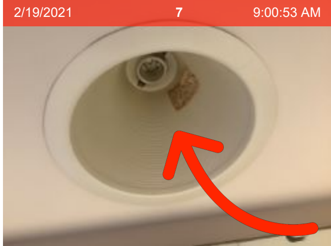
Light Fixtures | Bulb is missing
