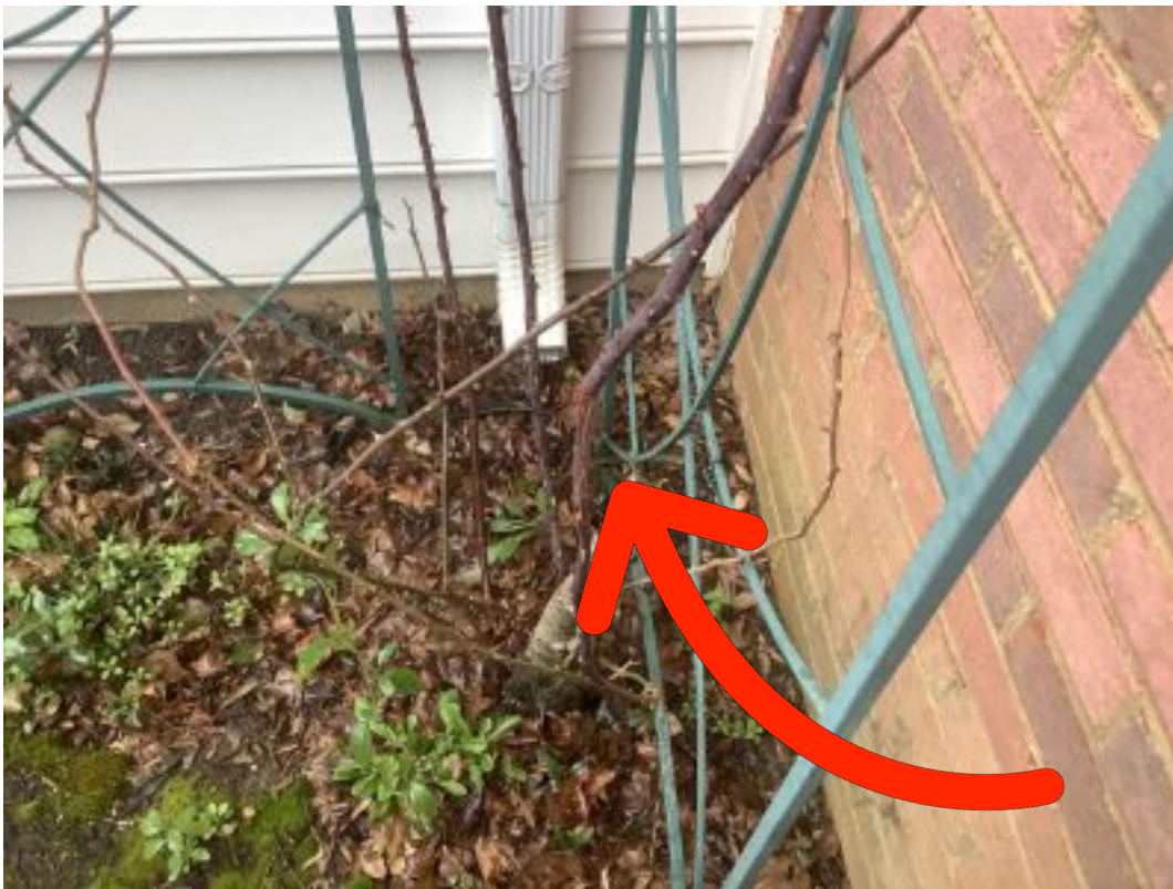
Front Exterior Downspout/Splash Blocks Splash block is missing.
