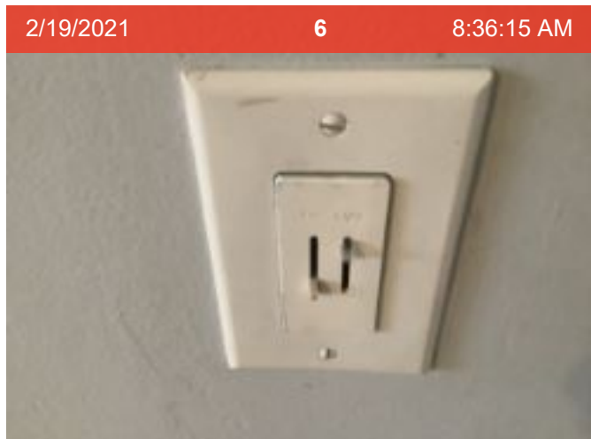
Outlet/Switch Covers | Knobs missing.
