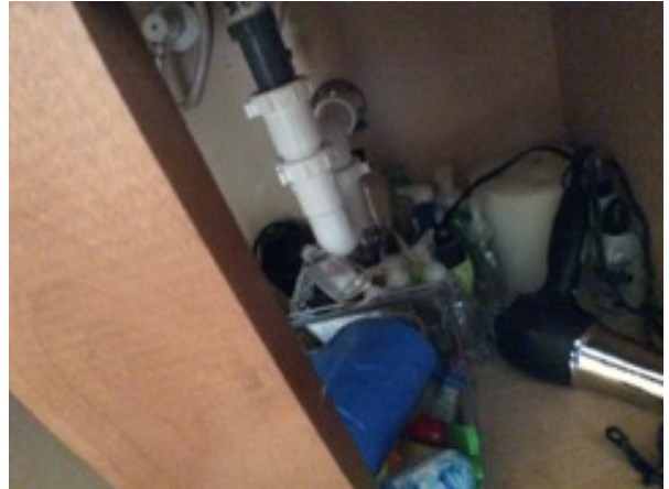
Cabinet Under Sink
