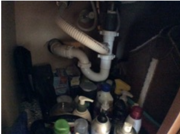
Cabinet Under Sink
