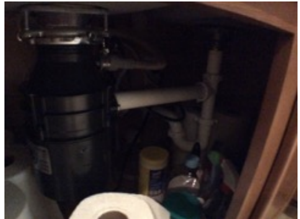
Cabinet Under Sink
