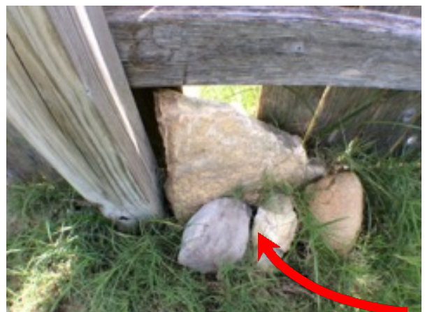
Fence - Broken slat.
