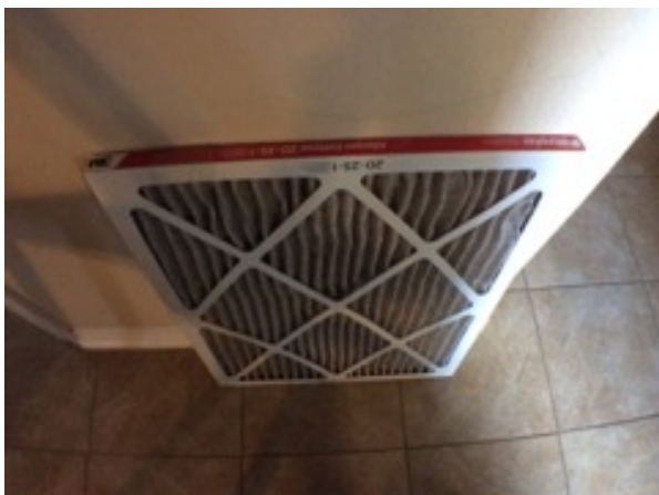
AC Filter - FILTER CONDITION: Filter recently replaced. Slightly dusty.
