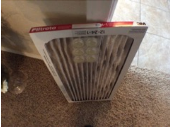
AC Filter 2 - FILTER CONDITION: Filter recently replaced. Slightly dusty.
