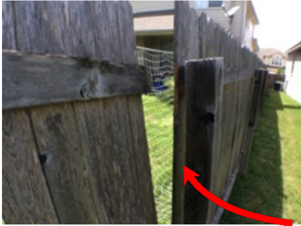
Fence - Section detached from fence post.
