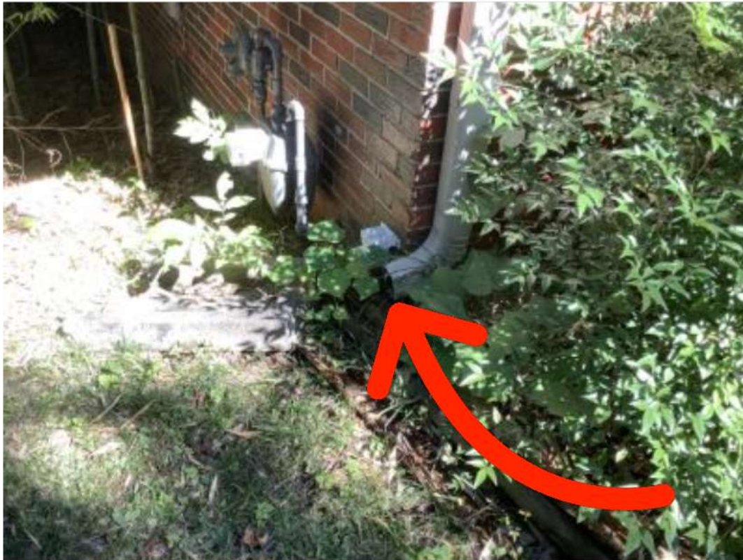
Front Exterior Downspout/Splash Blocks Splash guard moved
