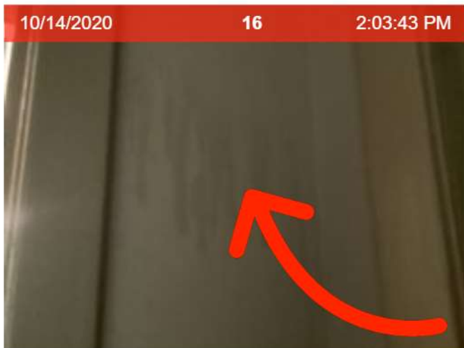
Walls/Paint | The wall is discolored
