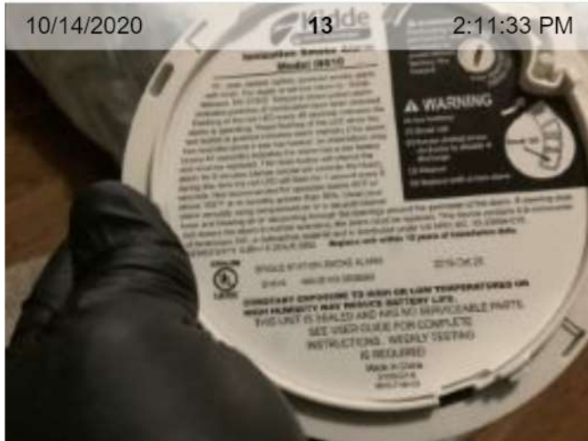
10/14/2020 13 2:11:33 PM Wireless Smoke Alarm Removed (mfd 10/2019) | Smoke test: Failed | Close-up of printed manufacture
