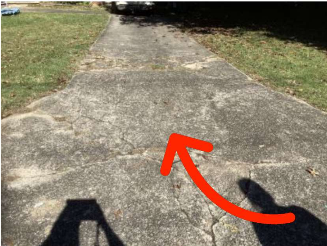
Front Exterior Driveway Major cracks in driveway
