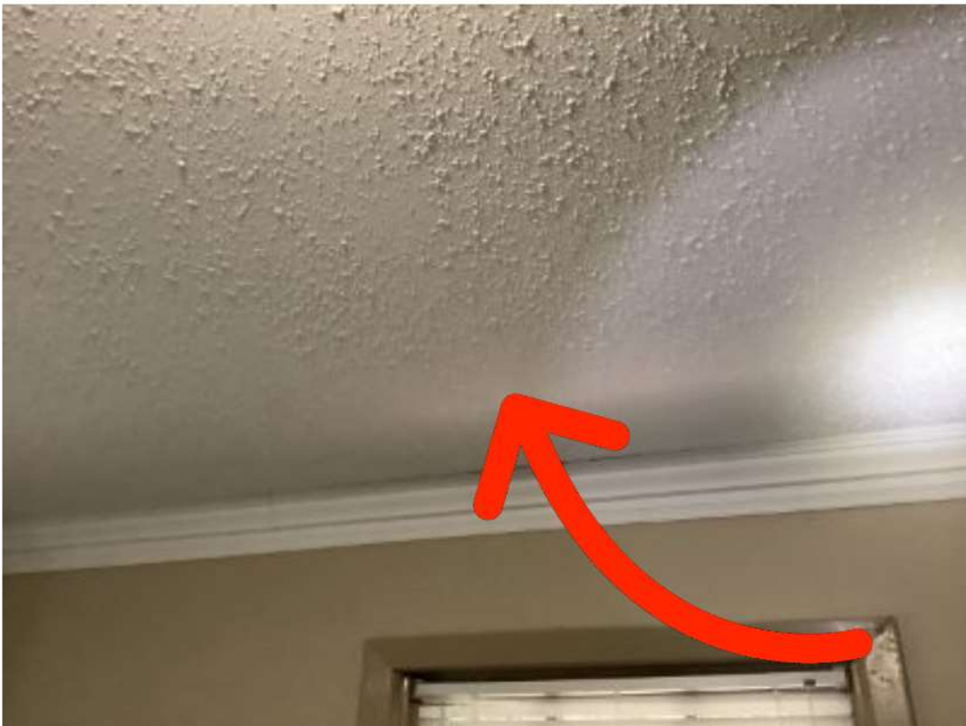
Bedroom 1 Ceiling Swag in ceiling
