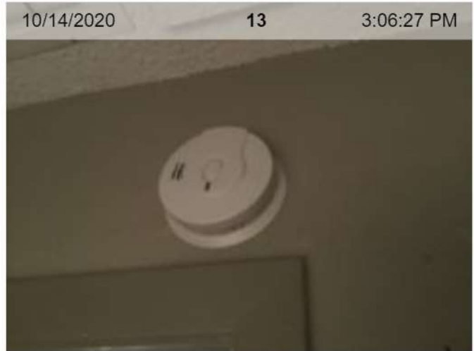
10/14/2020 13 3:06:27 PM Wireless Smoke Alarm Installed (mfd 5/2020) | Smoke test: Passed | Alarm in place (on ceiling or wall)
