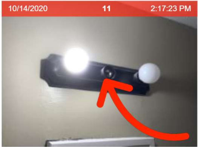
Light Fixtures | Bulb is missing
