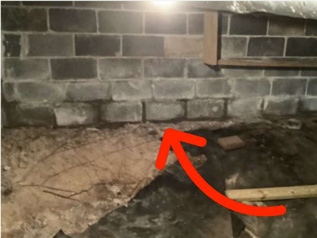
Basement Other Moisture present in basement
