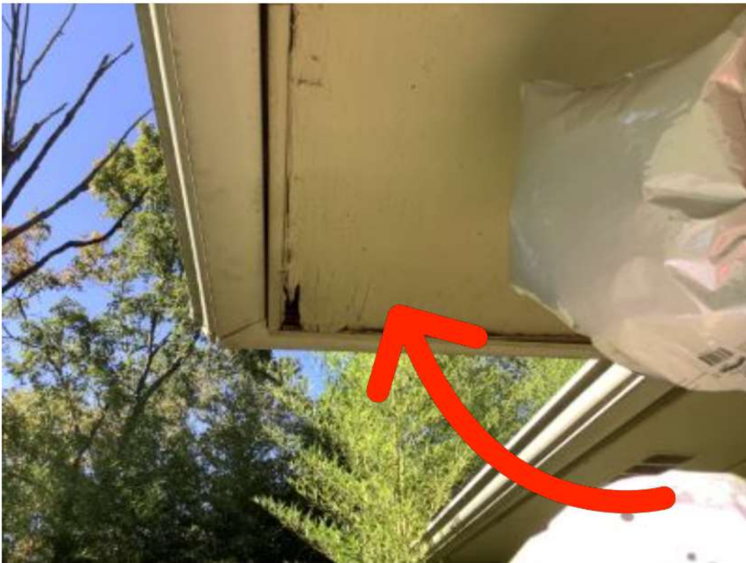
Entry Patio/Porch Rot on patio roof
