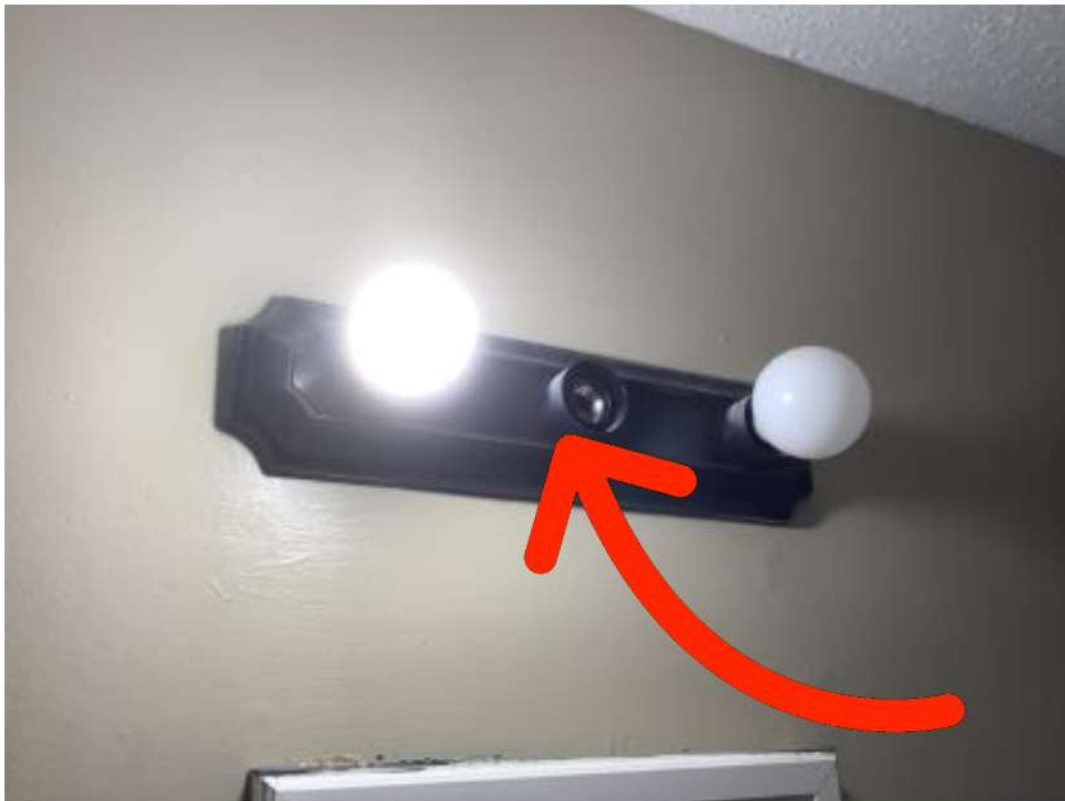
Bathroom 1 Light Fixtures Bulb is missing
