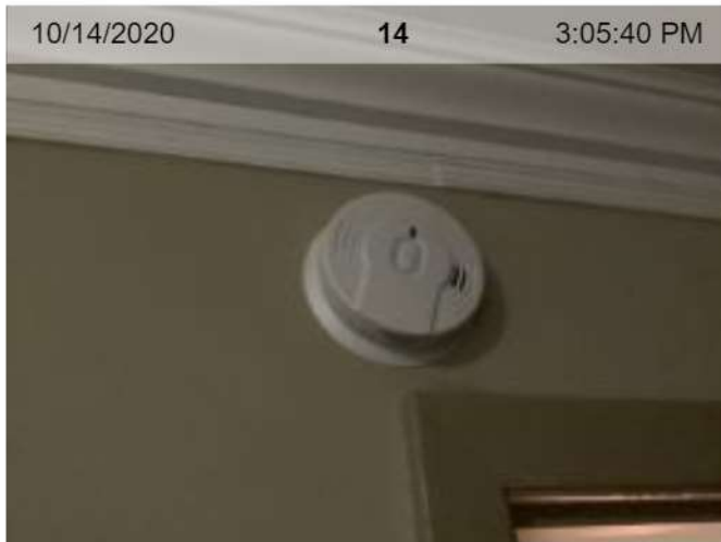
10/14/2020 14 3:05:40 PM Wireless Smoke Alarm Installed (mfd 5/2020) | Smoke test: Passed | Alarm in place (on ceiling or wall)
