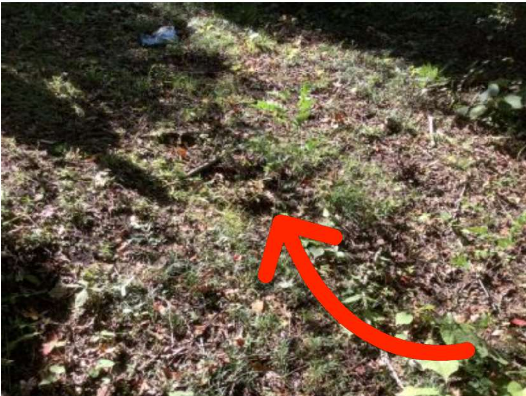
Rear Exterior Drainage Issues Right side of house
