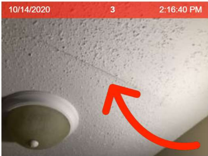
Ceiling | Cracks in ceiling showing signs of settling.
