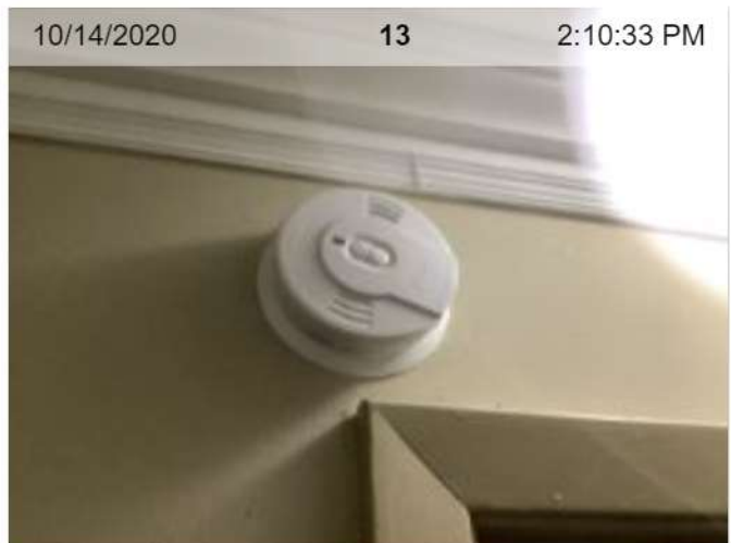
Wireless Smoke Alarm Removed (mfd 10/2019) | Smoke test: Failed
