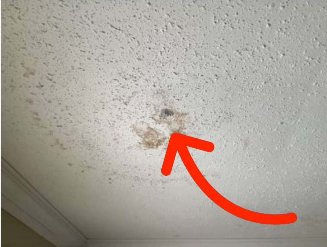
Living Room Ceiling The ceiling is discolored.
