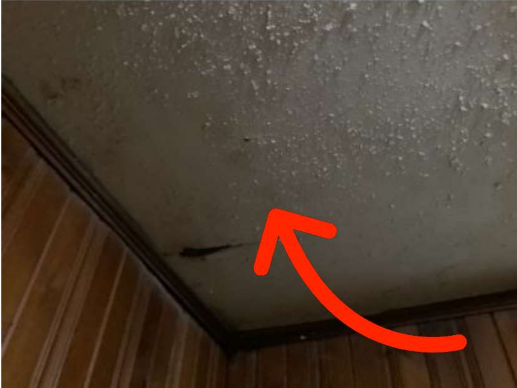
Bedroom 3 Ceiling Hole and bow in ceiling
