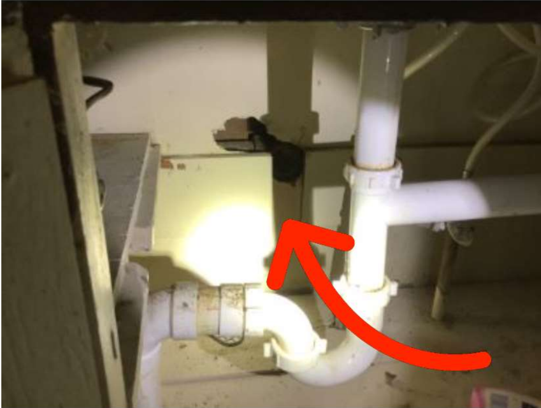
Kitchen Cabinet Under Sink Hole in back wall
