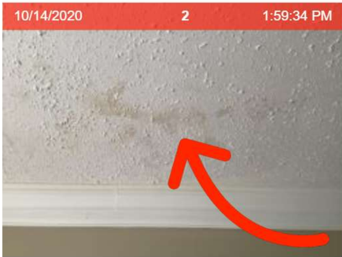
Ceiling | The ceiling is discolored.
