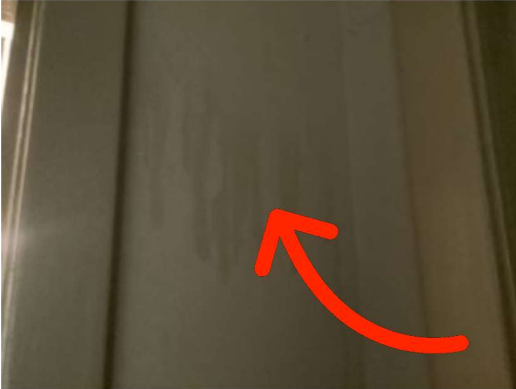
Hallway/Stairway Walls/Paint The wall is discolored
