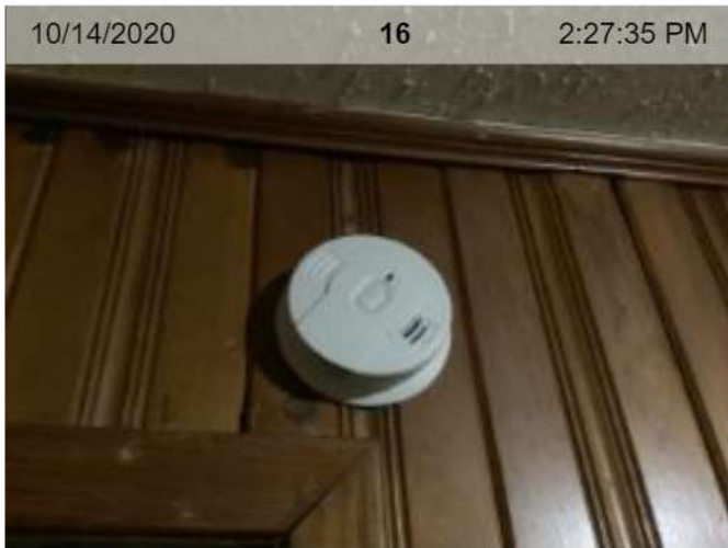
Wireless Smoke Alarm (mfd 10/2019) | Smoke test: Passed | Alarm in place (on ceiling or wall)
