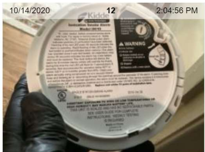
Wireless Smoke Alarm Removed (mfd 10/2019) | Smoke test: Failed | Close-up of printed manufacture
