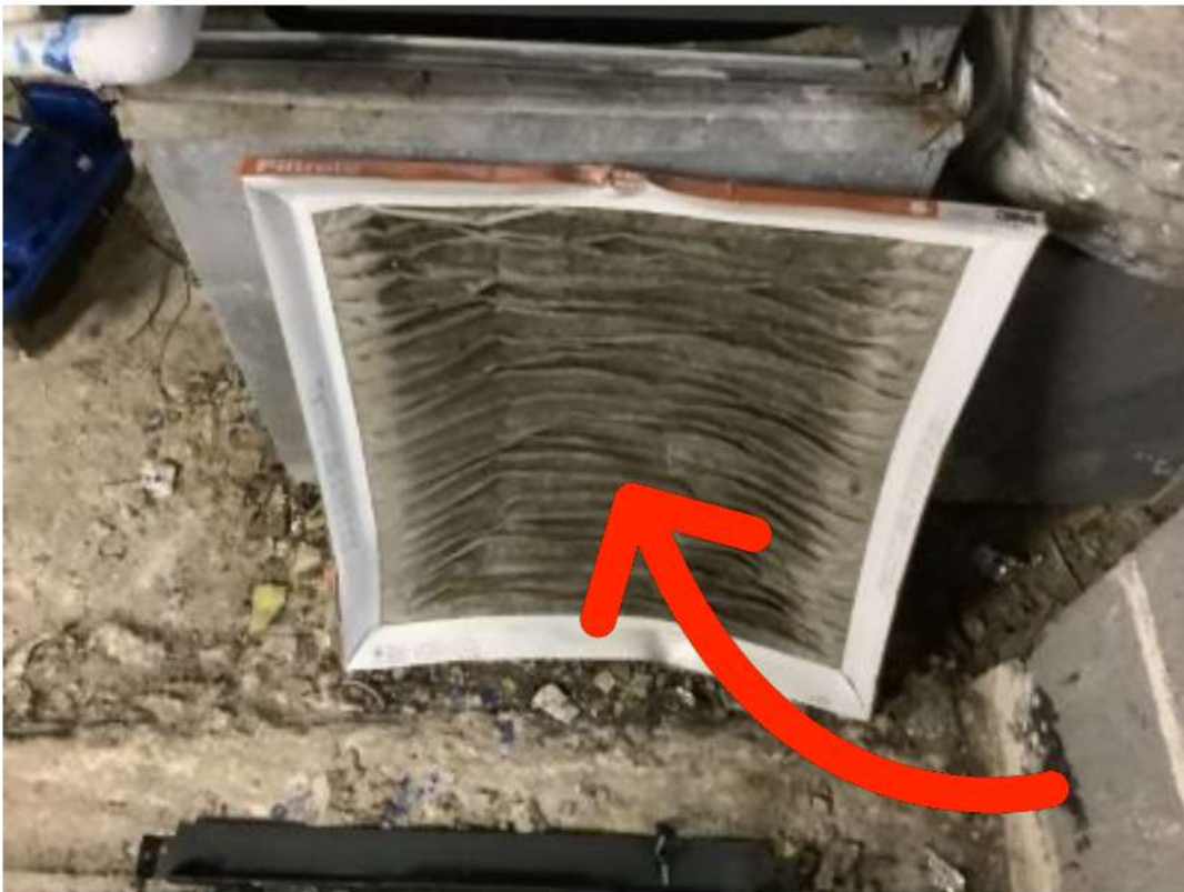
Basement Air Filter Back Wet
