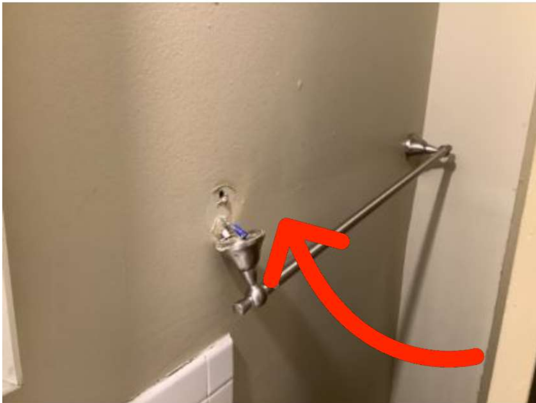
Bathroom 1 Towel Bars Towel bar is pulling away from the wall.
