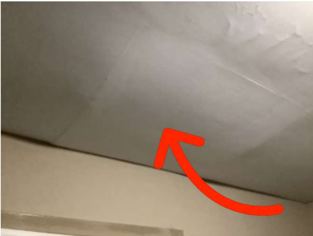
Bedroom 2 Ceiling Ceiling dropping down
