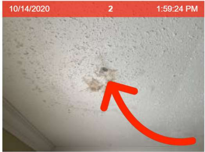
Ceiling | The ceiling is discolored.
