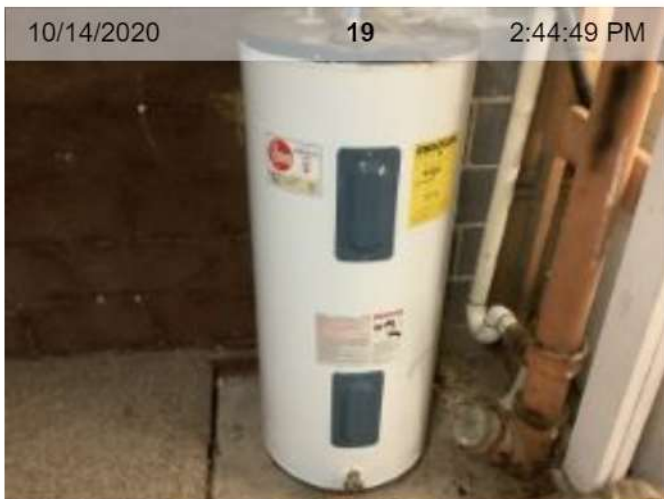
Electric Water Heater | >10 yrs old | Rheem | Water heater (with expansion tank if present)
