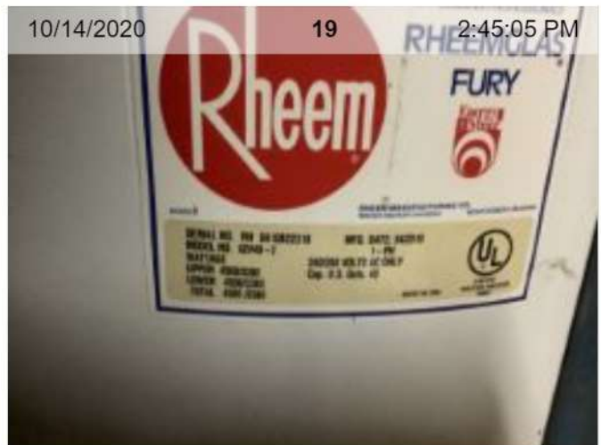
Electric Water Heater | >10 yrs old | Rheem | Water heater label
