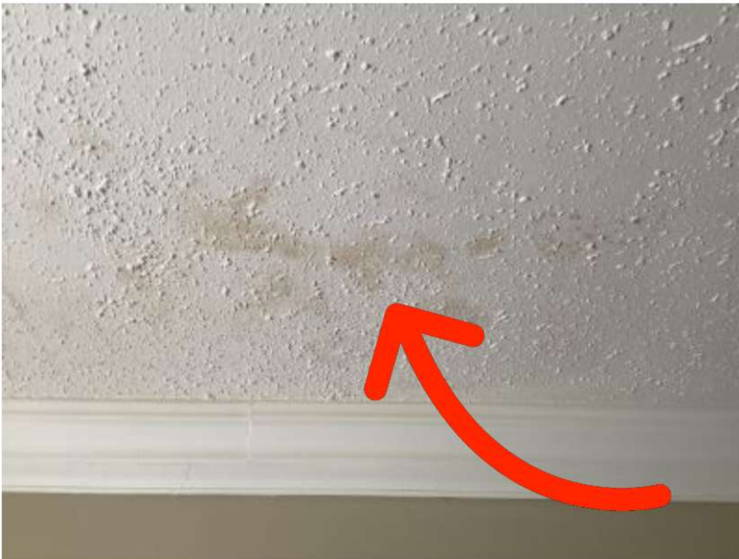
Living Room Ceiling The ceiling is discolored.
