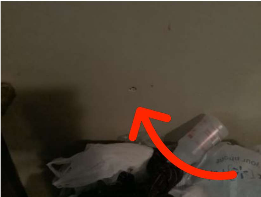
Kitchen Walls/Paint Holes in wall.
