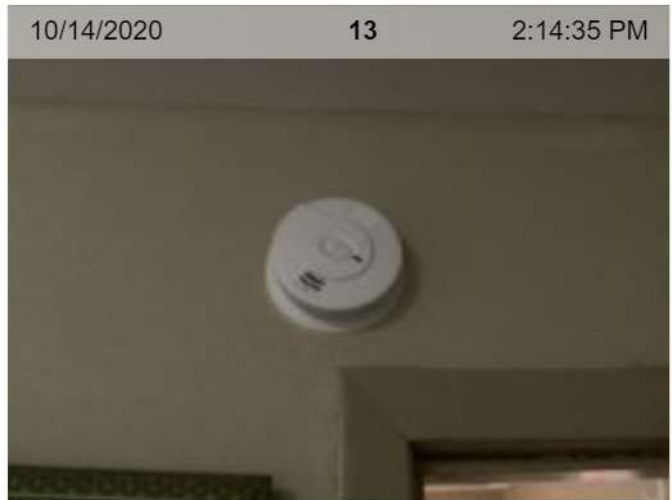
Wireless Smoke Alarm (mfd 10/2019) | Smoke test: Passed
