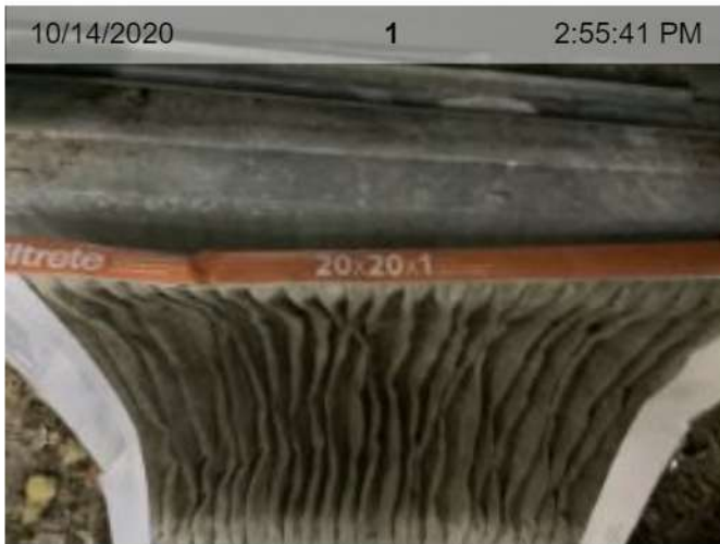
20 x 20 x 1 Air Filter Removed | Close-up of size/initials/date
