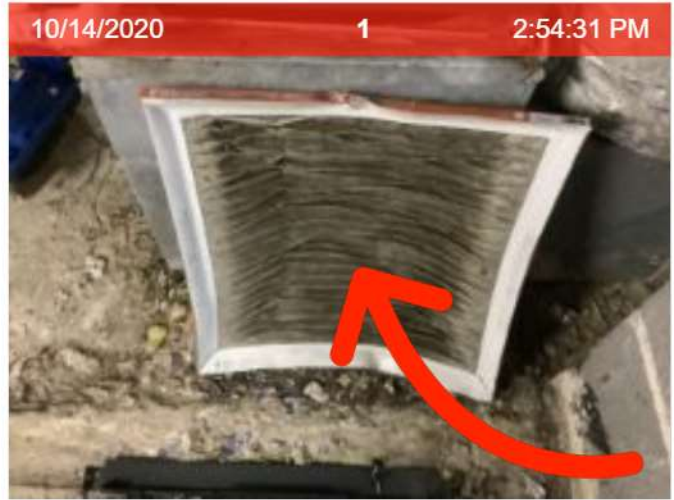
20 x 20 x 1 Air Filter Removed | Back
