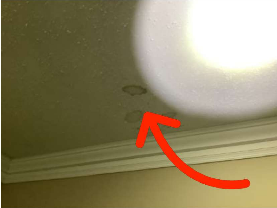
Bedroom 1 Ceiling The ceiling is discolored.
