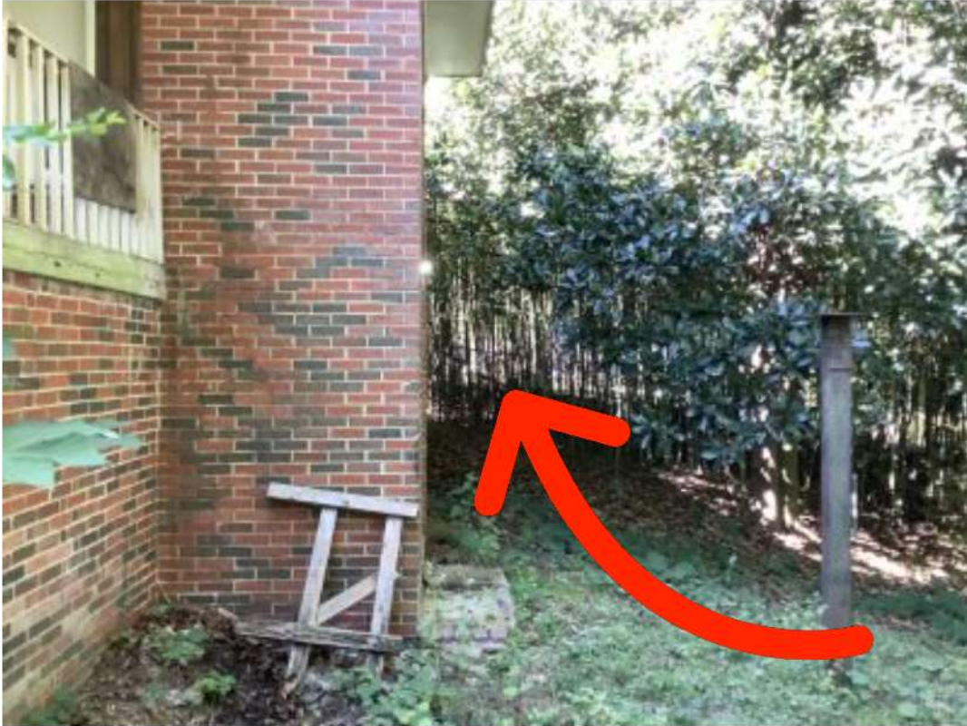
Rear Exterior Porch/Patio/Deck Deck missing
