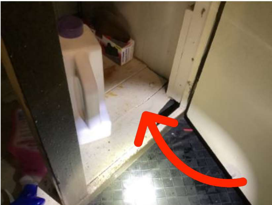
Kitchen Cabinet Under Sink Hole in base
