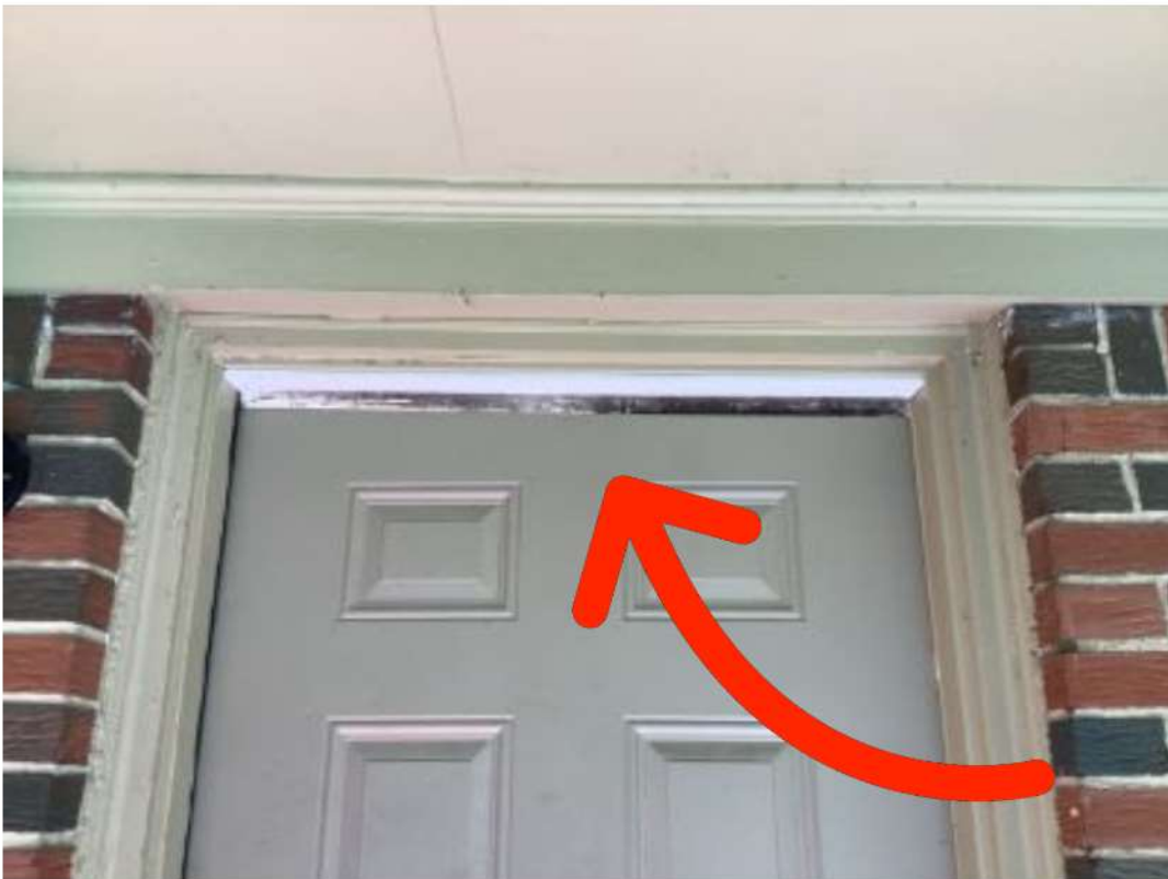
Entry Front Door Exterior Discoloring on trim
