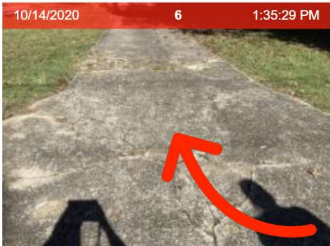
Driveway | Major cracks in driveway
