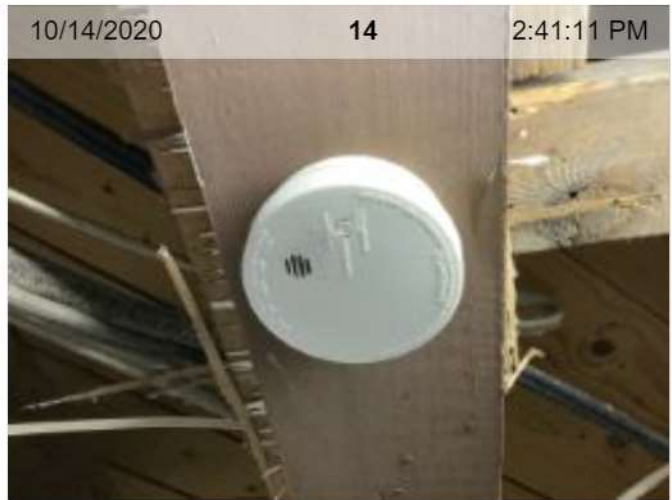
Wireless Smoke Alarm Removed (mfd 10/2014) | Smoke test: Failed | Alarm in place (on ceiling or wall)
