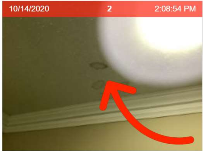
Ceiling | The ceiling is discolored.
