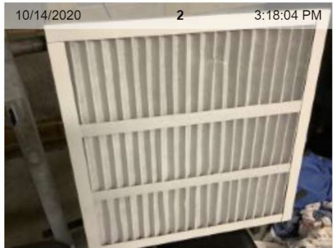
20 x 20 x 1 Air Filter Installed | Front
