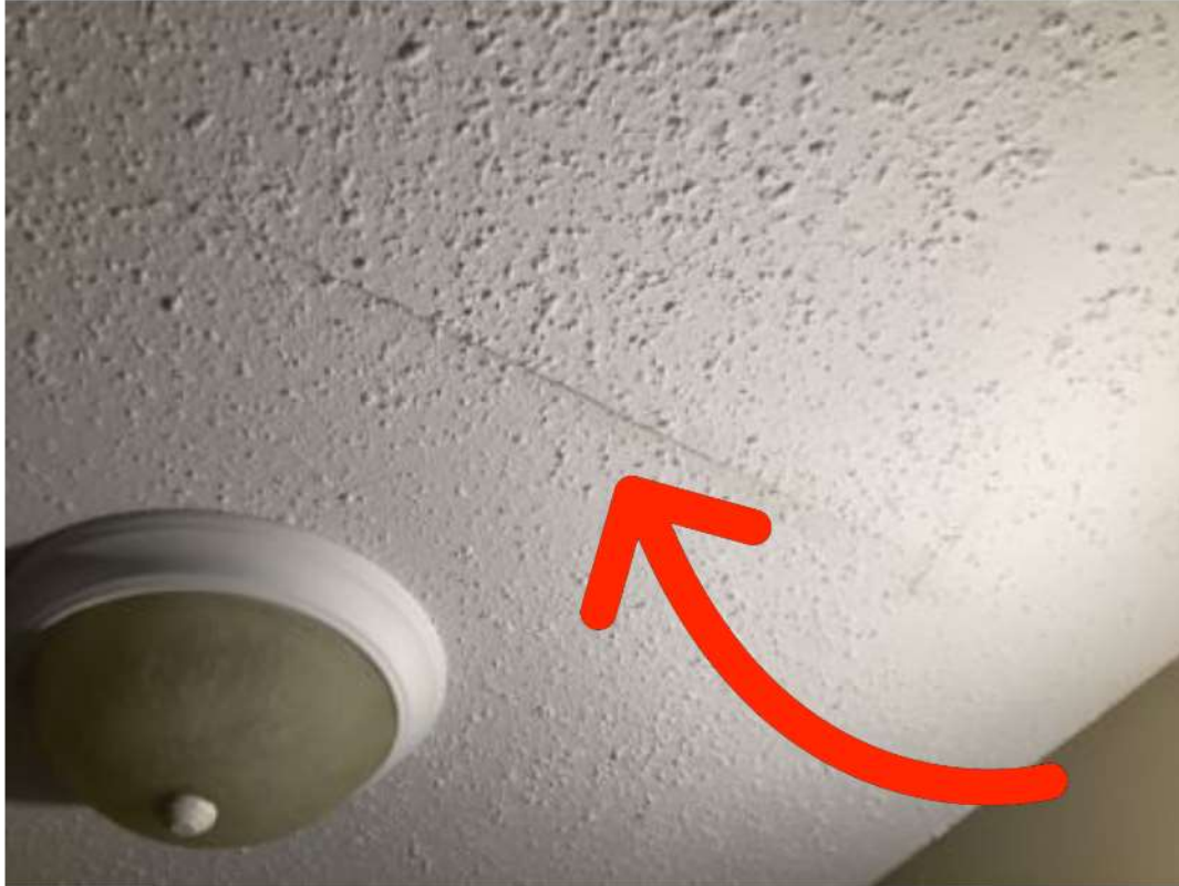
Bathroom 1 Ceiling Cracks in ceiling showing signs of settling.
